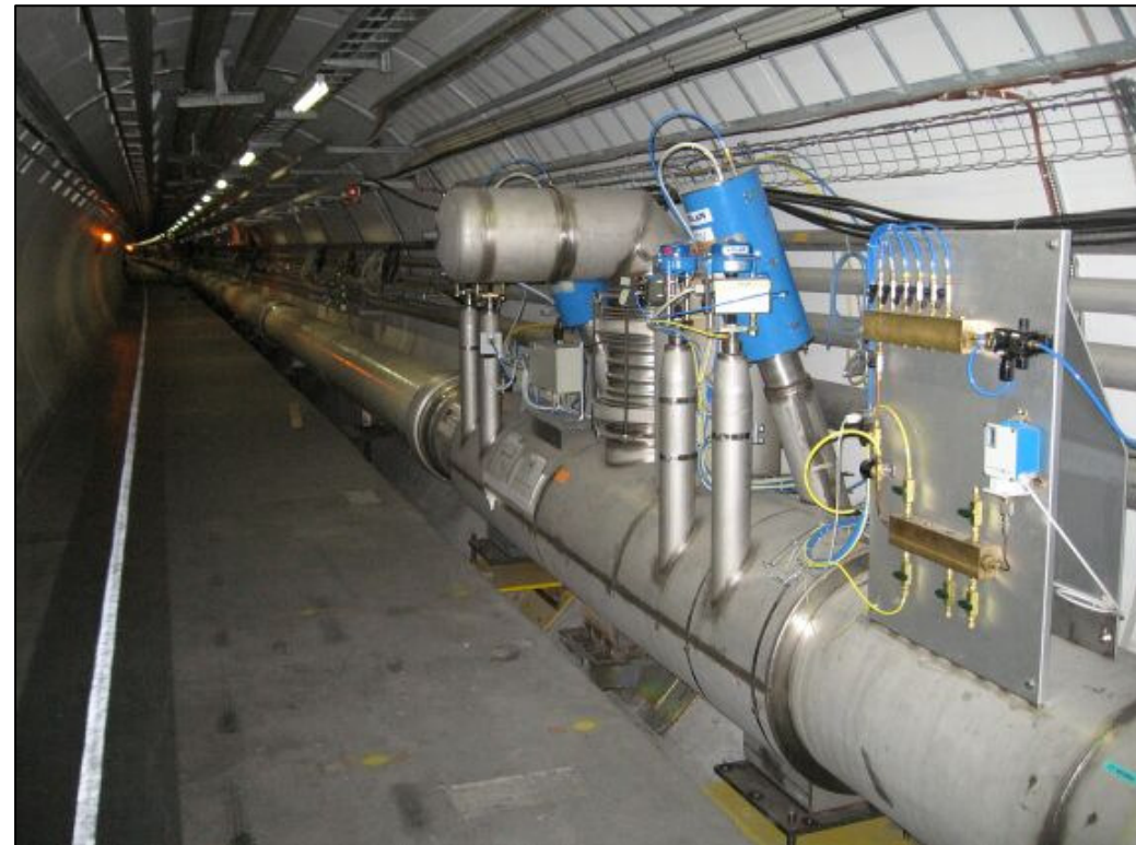
The LHC Cryogenic Distribution Line during the reception tests in sector 8-1
